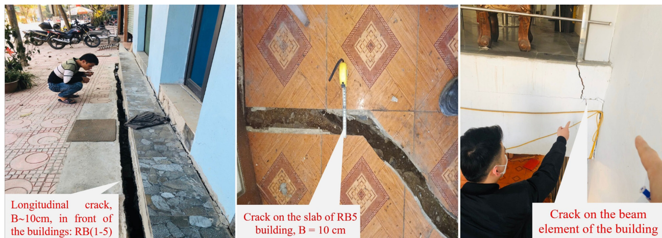
Figure 8. Extensive damage to the residential buildings located on the study slope.
