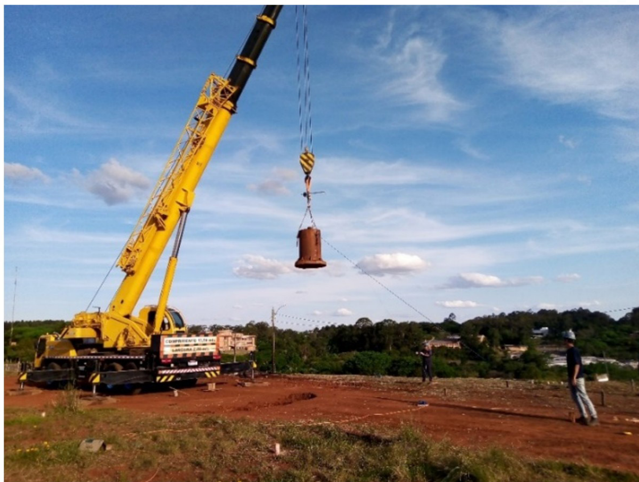
Figure 14. Field opening verification test.
