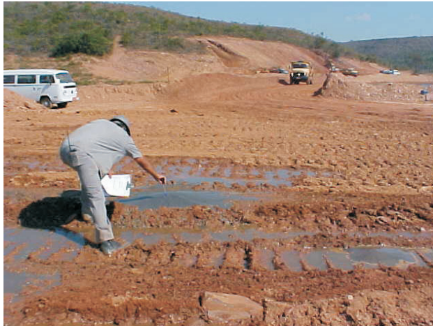
Figure 18 - Sand boils on the top of the first embankment layer.
