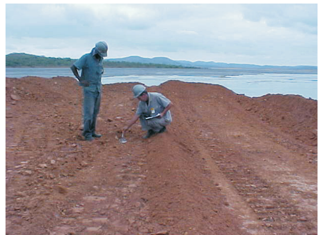
Figure 17 - Sand boils on the top of the first layer.
